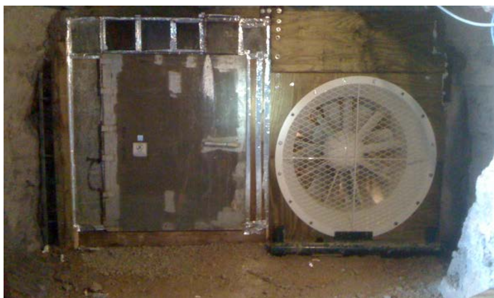
Figure 7.18. East booster fan installed in bulkhead
